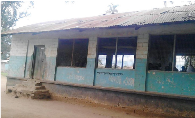
Mwembesongo primary school - renovations (Before)
