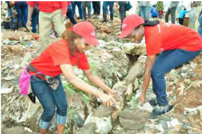
Jubilee Insurance members of staff join volunteers at Shafco primary school in Mathare North slum where they helped in construction of gabions, cleaning and painting.
