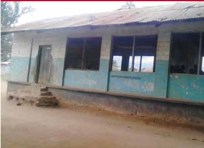
MWEMBESONGO PRIMARY SCHOOL - RENOVATIONS (BEFORE)
